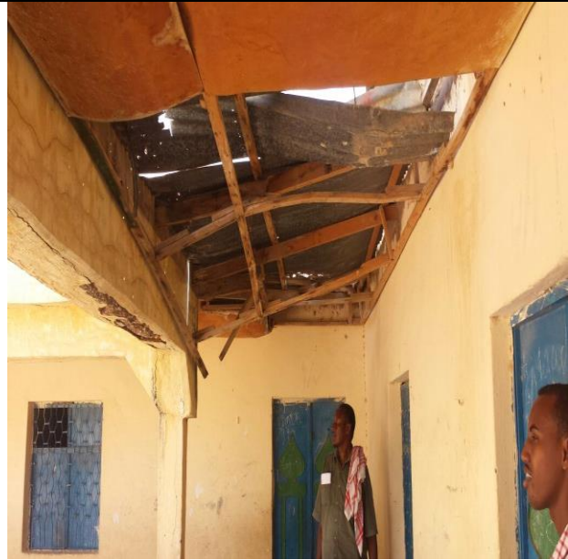
Broken ceils and the roof of Daru-Salam primary school
