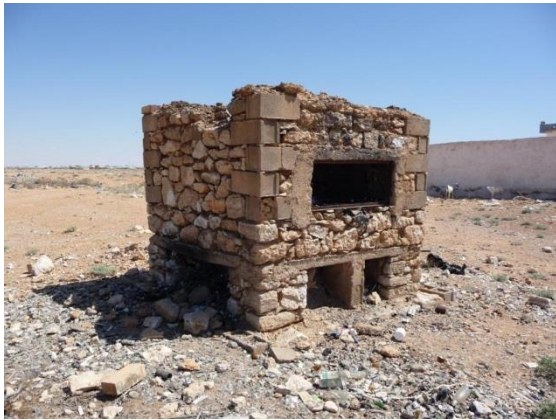
Plate 9 The medical waste incinerators at the main hospital no longer function due to a lack of maintenance. Such costing must be budgeted into hospital running costs and not neglected
