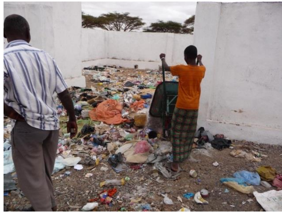
Plate 12 Newly constructed waste transfer station being used inappropriately by a local youth. Dumping the waste in the entrance will soon block access.
